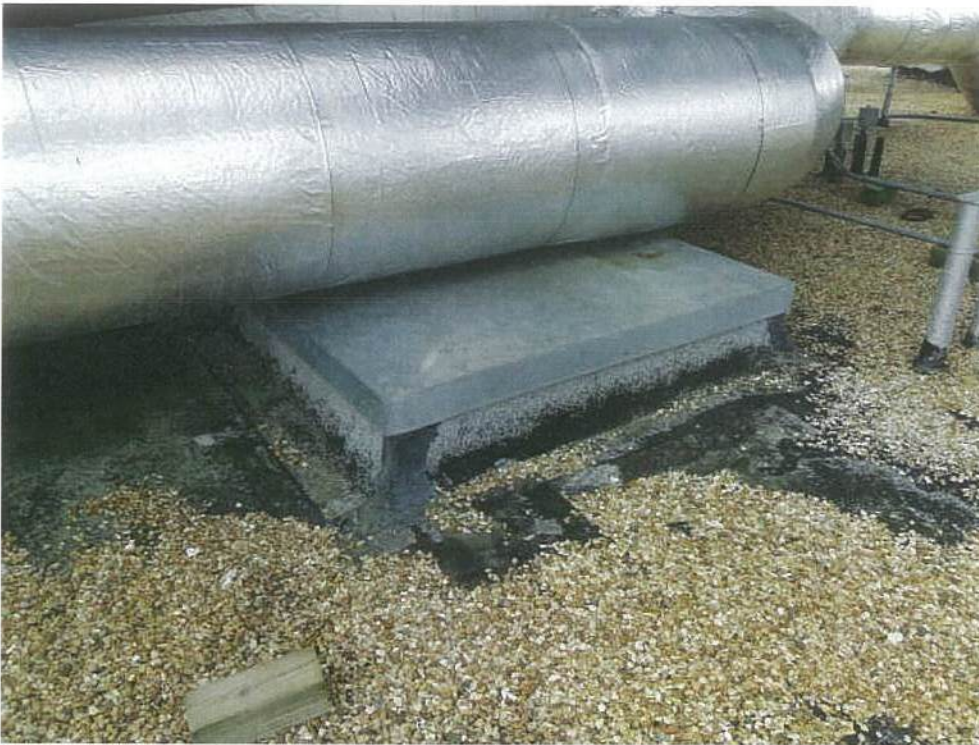
Photo #5 View of abandoned equipment curb to be removed and roof deck opening closed at Roof Area 1. Provide Miro Model #8-DS-SB duct support as shown below.
