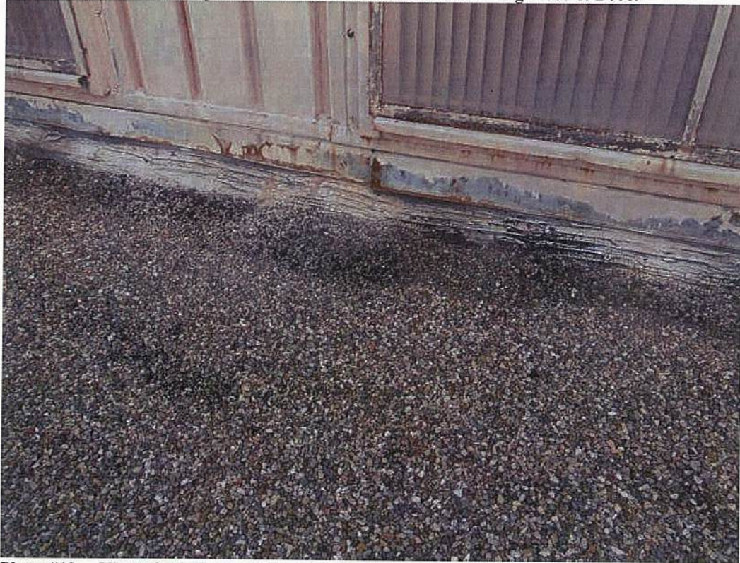
Photo #12 View of existing metal counter flashing at Bldg. B006 offset wall.
