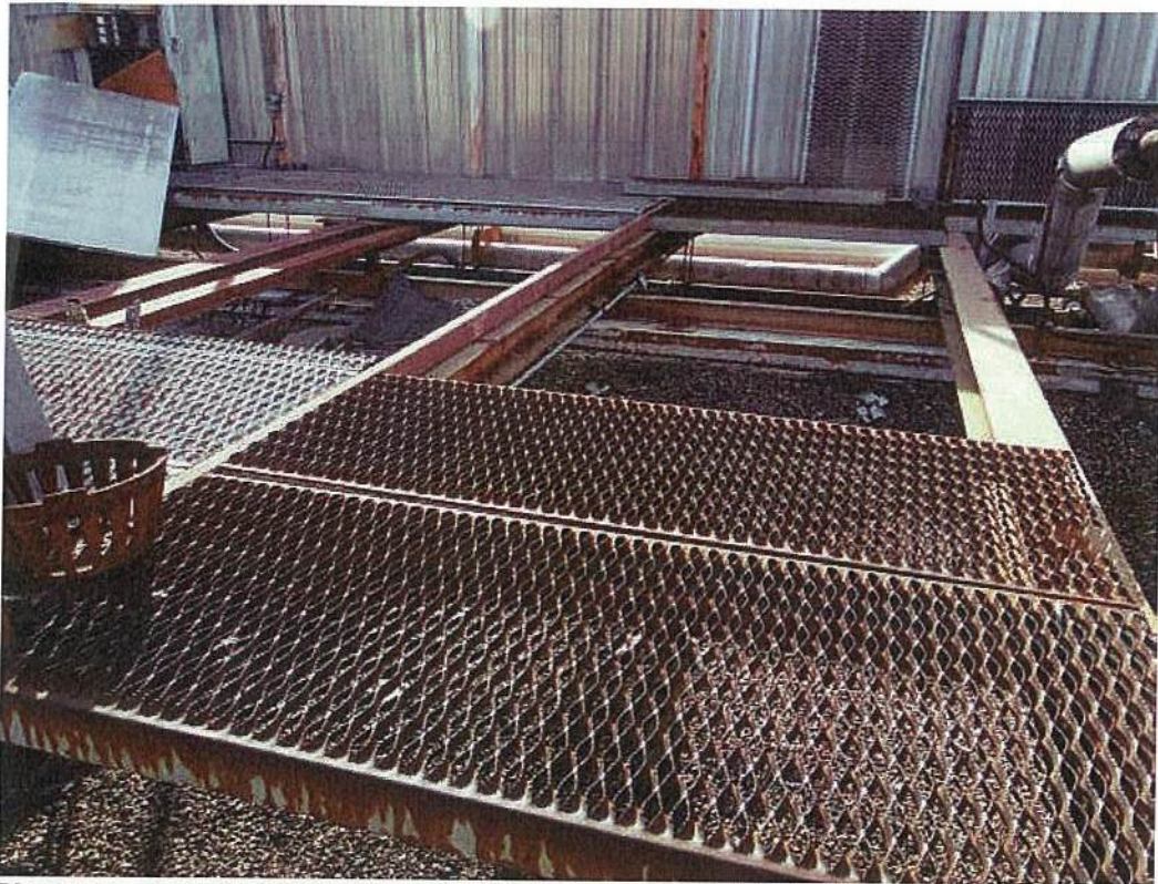
Photo #11 View of steel platform scheduled to be removed at Bldg. B005 & B006.
