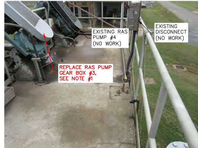
B 5 PHOTO @ RAS PUMP (LOOKING SOUTH)
