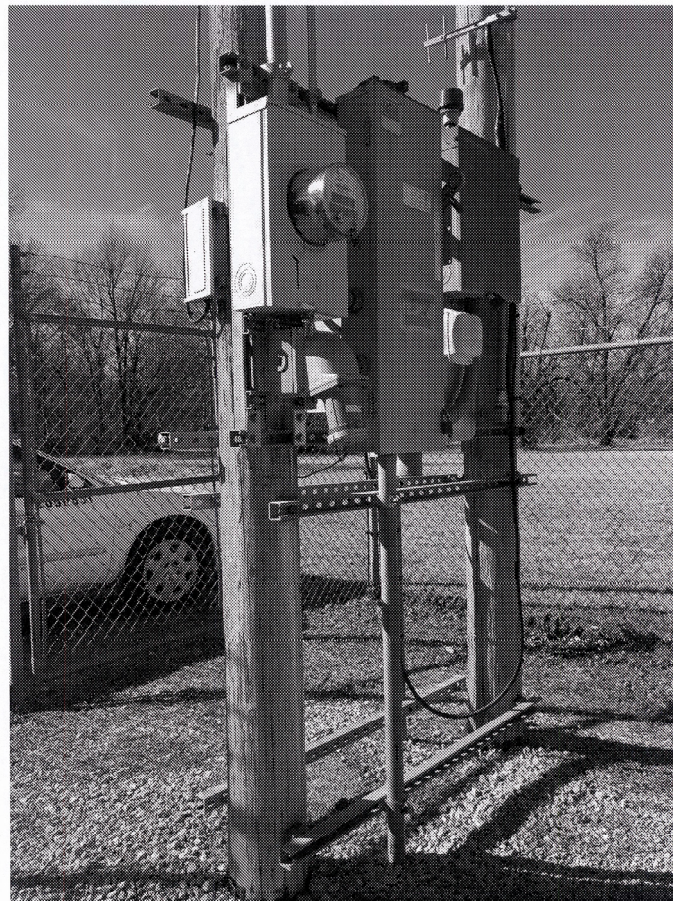
3 PHOTO — EXISTING ELECTRICAL SERVI 18 NTS
