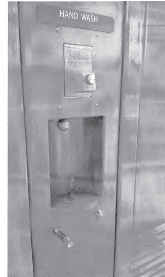
HAND WASH STATION
