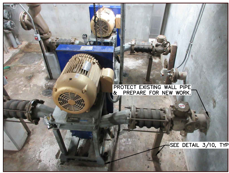
A EXISTING TWAS PUMPS PHOTO 4 NTS
