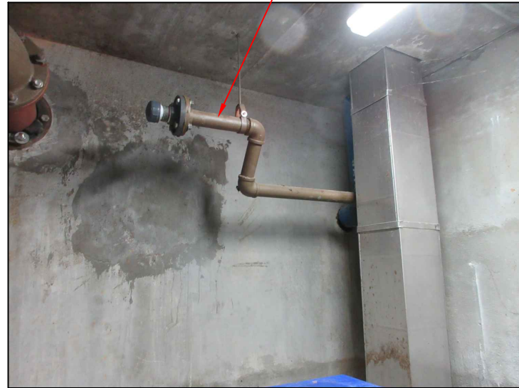
A 8 NTS PRESSURE VALVE & PIPING PHOTO
